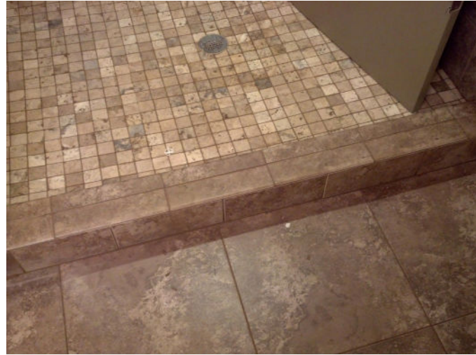
Increased chance of leaks, mold and mildew
